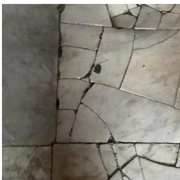
Fig. 5: Damaged marble floor Photo: iefimerida.gr
